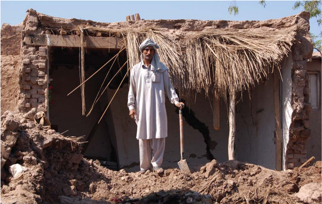
Damage caused by floods in Pakistan in 2010.
